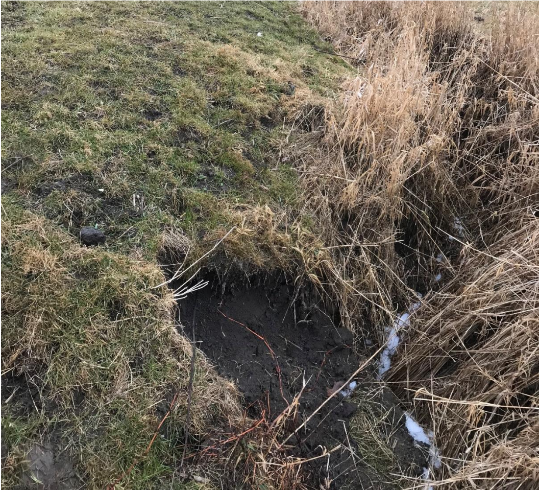
Image 8.0 – Chute 8: Severe undercut with slump and vegetative overhang
