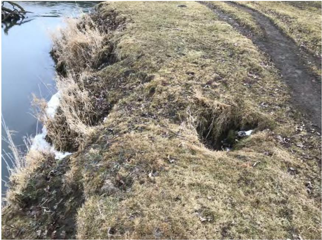
Image 7.0 – Chute 7: Moderate undercut with slump and vegetative overhang
