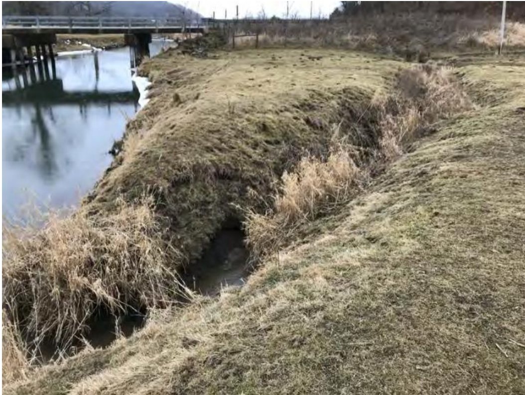
Image 8.1 – Chute 8: Severe undercut with slump and vegetative overhang
