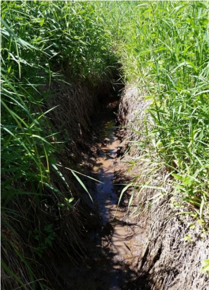
Image 1.0 – Chute 1: Severe undercut with bare banks and vegetative overhang
