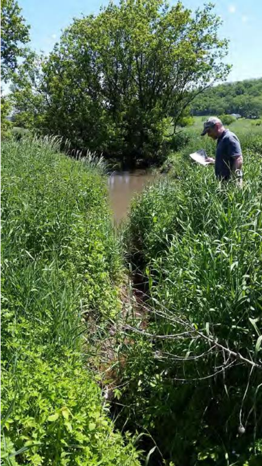
Image 2.0 – Chute 2: Moderate undercut with vegetative overhang
