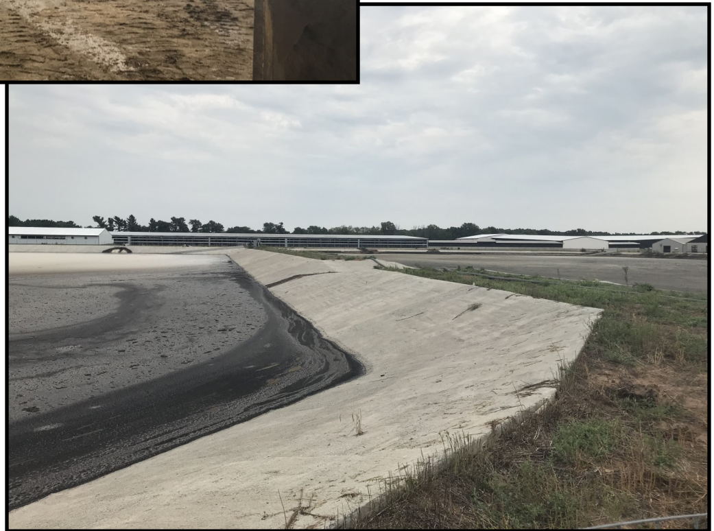
Photo 11 (right): Looking east at the overflow channel between WSF 1 and WSF 2. The channel was clear of manure and other debris.
