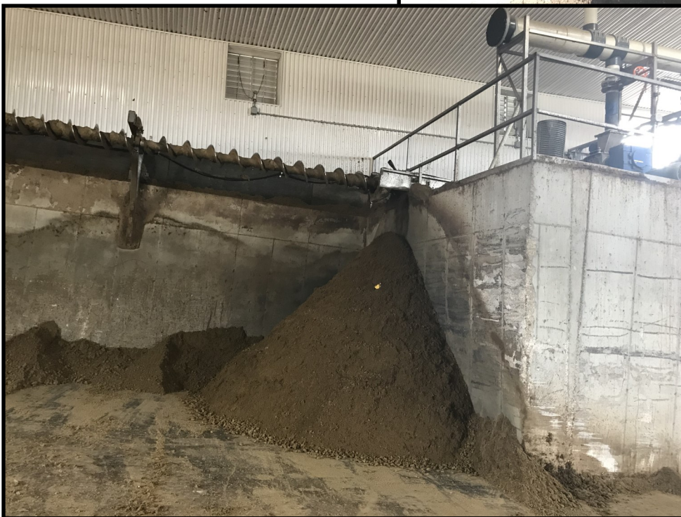
Photo 9 (bottom left): Looking within the solid manure separation building. Separated manure solids are staged within the building and are returned to the barns to be used for bedding. A proposed expansion to the building will include the installation of dryer to further dry out manure solids prior to being brought back to the barns.
