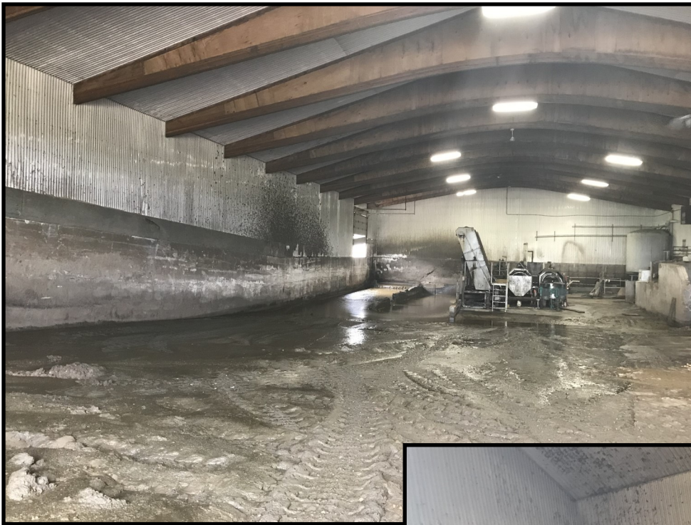
Photo 7 (top left): Looking at the waste transfer lanes within the sand separation building. The operation no longer uses sand bedding, however, the transfer system within the building is still in use.
