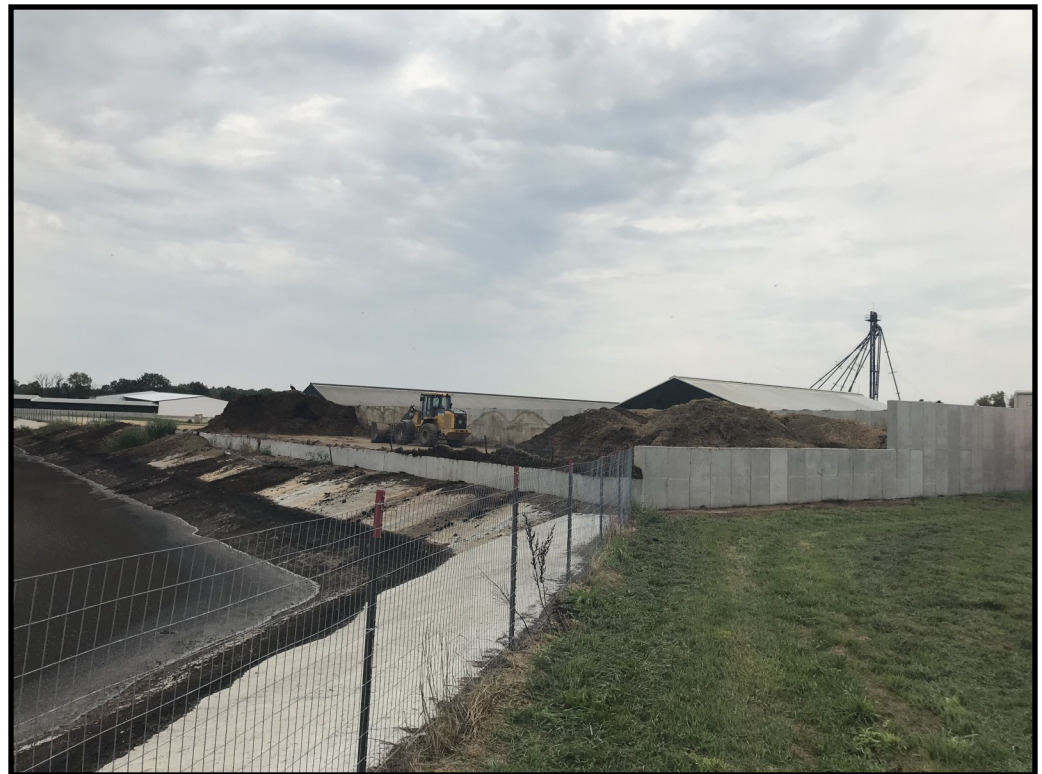
Photo 13 (right): Looking east toward the solid manure stacking pad at the south west corner of WSF 1. The concrete walls around the perimeter contain material within the stacking pad boundaries. Leachate and runoff from the stacking pad flows directly into WSF 1.
