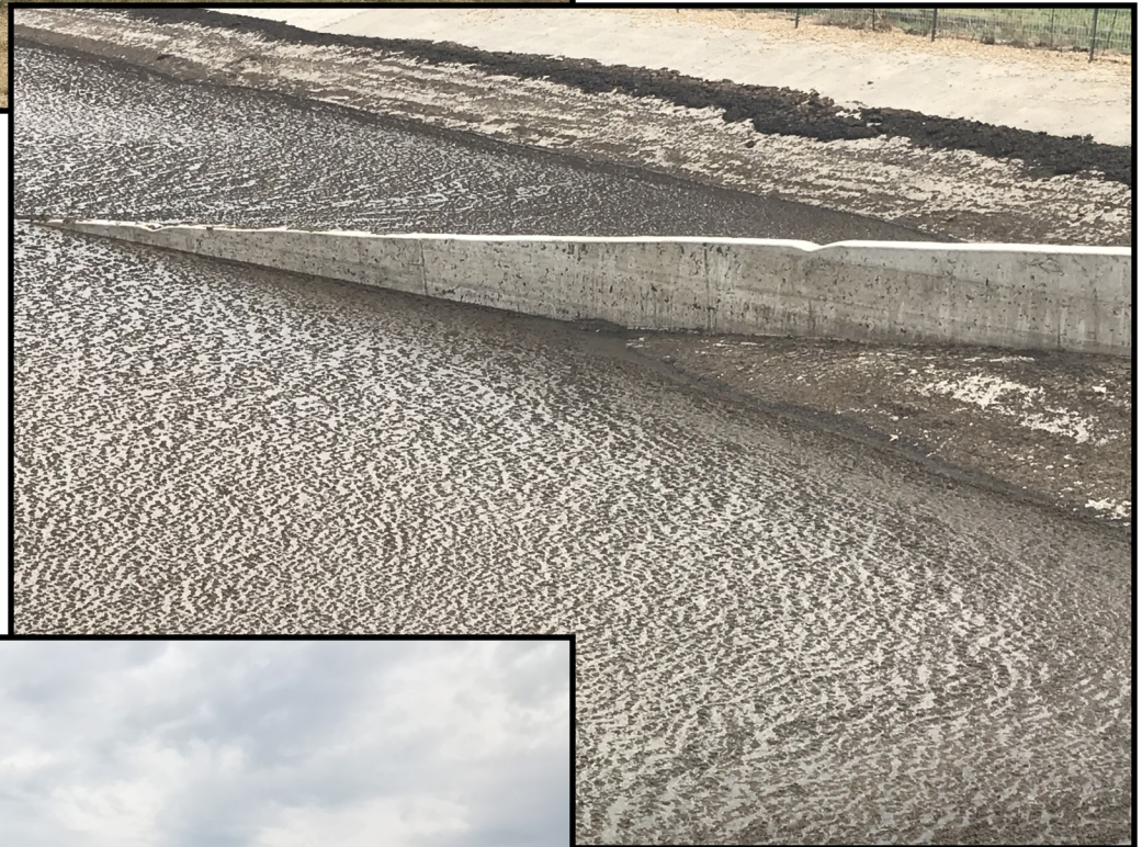
Photo 3 (right): Looking at the concrete ramp within WSF 1. Notches which serve as permanent markers can be seen within the concrete.
