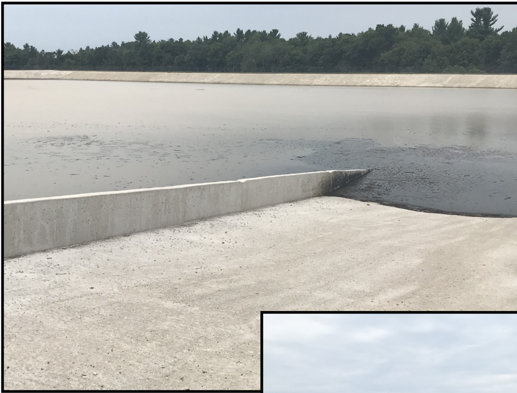
Photo 5 (left): Looking north from the south east corner of WSF 2. Notches which serve as permanent markers can be seen on the concrete ramp. A safety fence was also observed around the entire perimeter of the storage facility.
