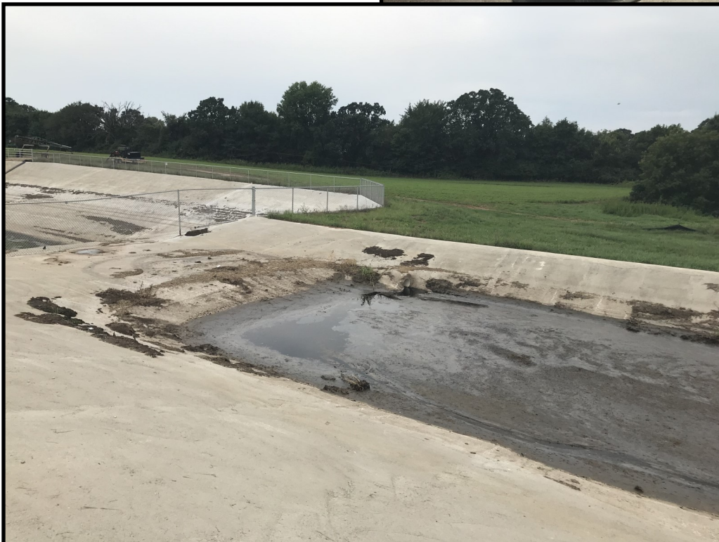
Photo 20 (bottom left): Looking west at the end of the concrete transfer swale pictured in photo 18 where leachate and feed storage runoff enter the process wastewater storage facility.
