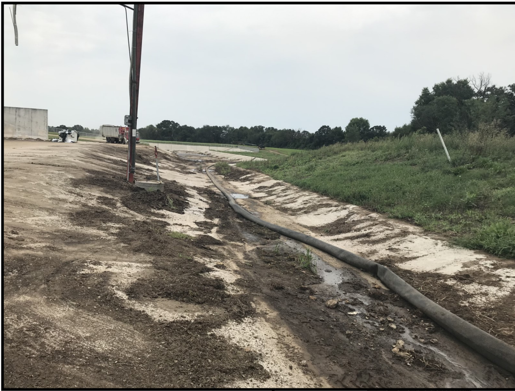
Photo 18 (top left): Looking south down the concrete transfer swale that directs leachate and feed storage runoff into the process wastewater storage facility.
