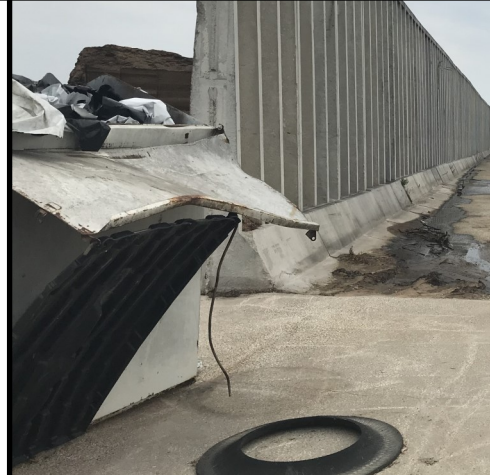
Photo 19 (right): Looking east down the concrete transfer swale which directs leachate and feed storage runoff from the east portion of the feed storage into the transfer swale pictured in photo 18.
