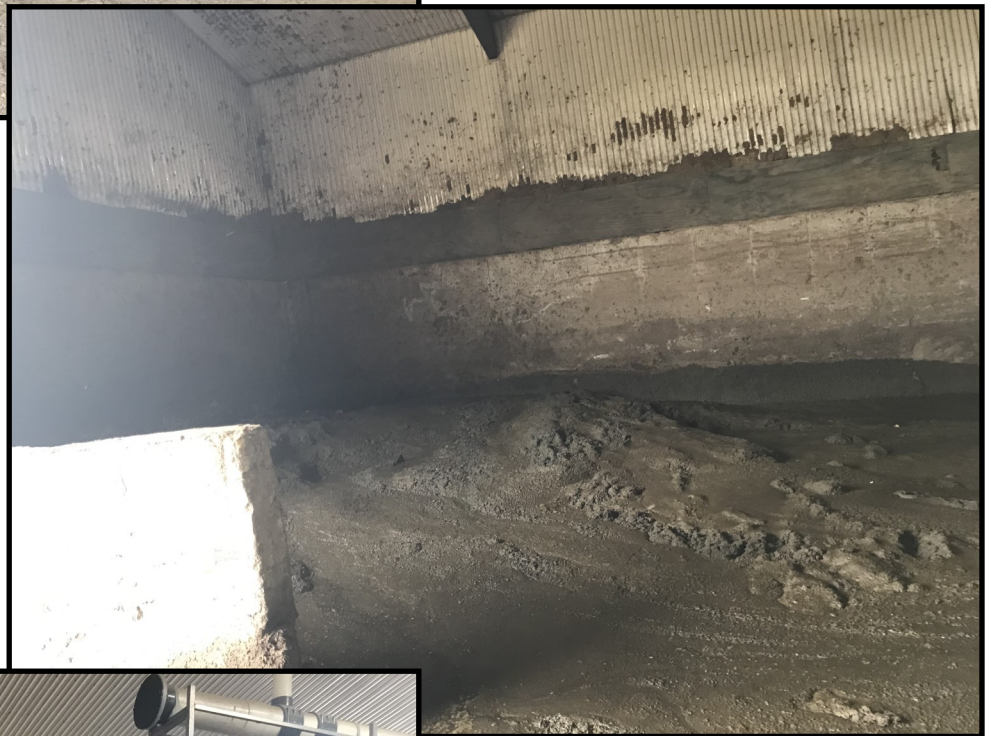
Photo 8 (right): Looking at a manure laden sand pile within the sand separation building. Sand is still being flushed out of the manure transfer system since the operation discontinued use of sand bedding. Manure laden sand that is flushed out is piled above the transfer lanes (pictured in photo 7) to allow liquids to drain out prior to being land applied or brought to solid manure storage.
