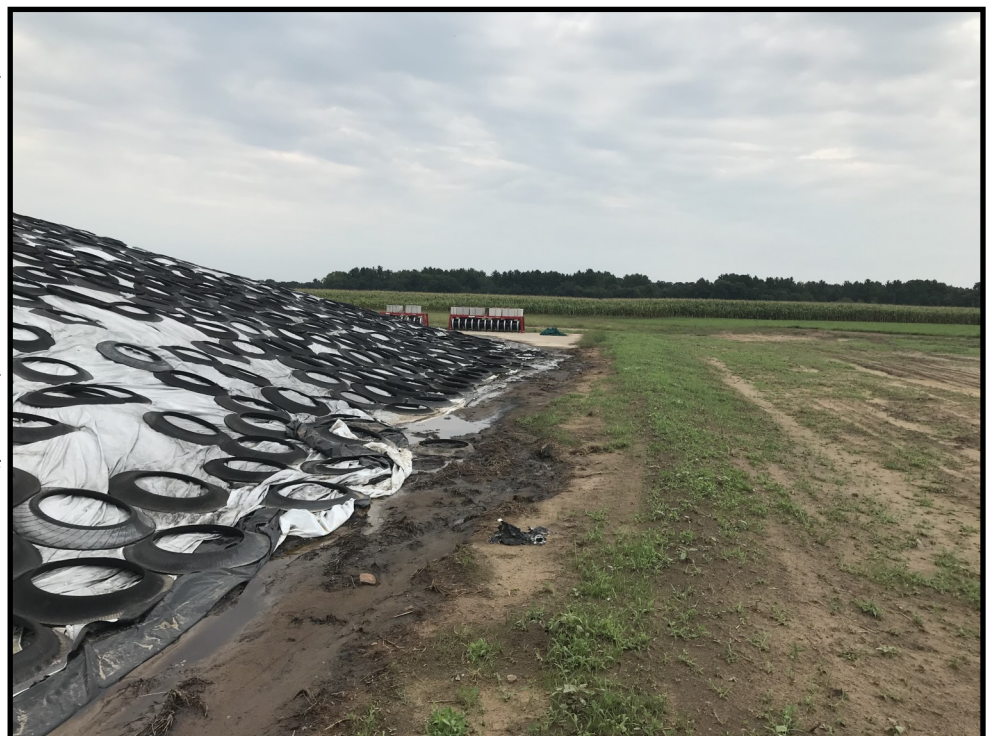
Photo 17 (right): Looking east along the southern edge of the feed storage area. Dark liquid can be seen along this edge of the feed storage.
