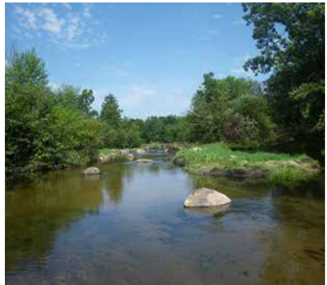
Upper Tomorrow River: boulder retard placement, wing deflector on right, LUNKER installation upstream left
