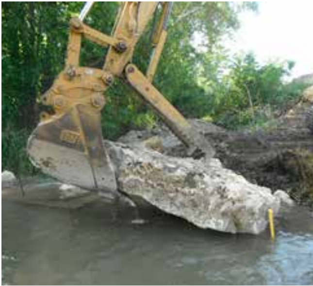
Placing the first, large "face rock" onto a series of three LUNKERS structures.
