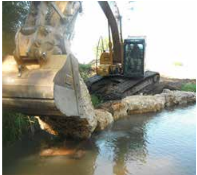
Placing the last "face rock" onto the same series of three LUNKERS structures.
