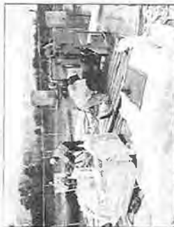
Work on the dam at McDill Pond is expected to be completed by the end of the year. (A.C. News Staff / Journal Staff)
