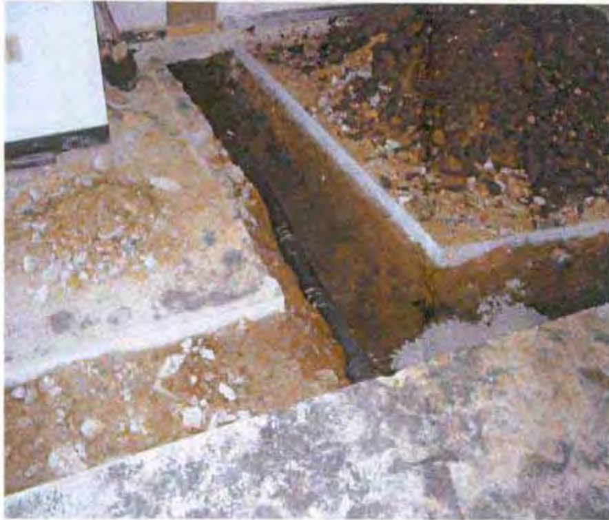
5. General view of 4" perforated pipe within the trench. This is the new extraction pipe for the sub-floor vapor mitigation system.
