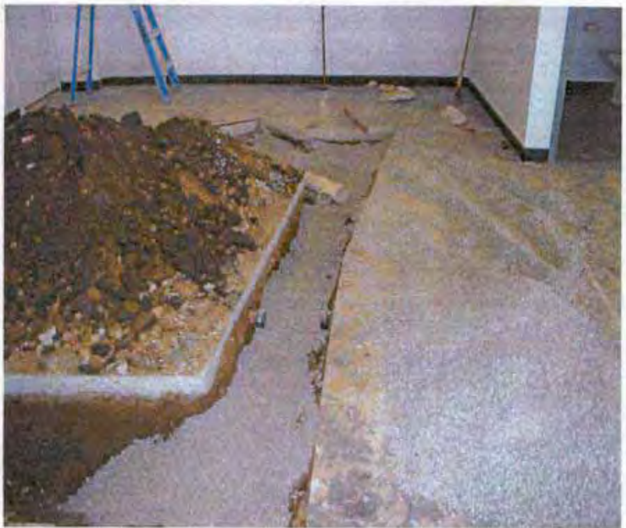
6. The placement of pea gravel on top of the sub-floor vapor mitigation extraction pipe. Floor drain piping lying on top of the gravel.
